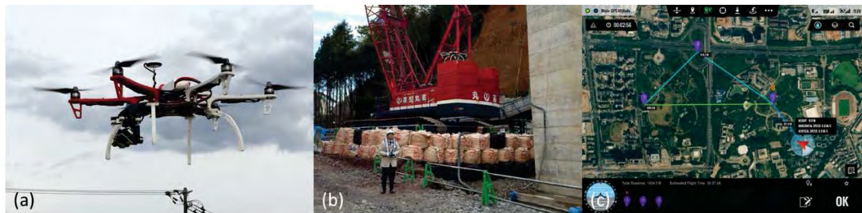
Figure 2. (a) camera-equipped UAV (b) operator executing data collection task on the construction site, (c) waypoints setting in commercially available application (DJI Ground Station 2015).
